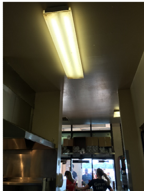
Interior fluorescent lighting.
