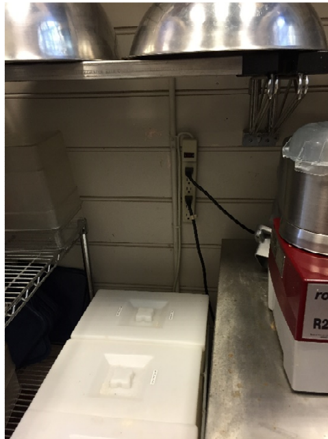
Existing plug strips.
