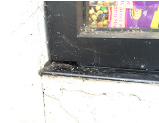
No sealant at frame.
