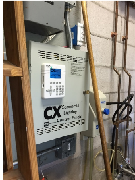
Lighting Control system
