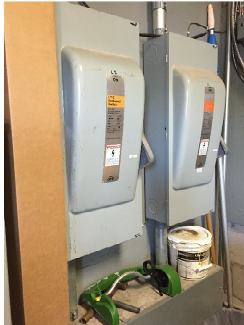
(2) 200A fused disconnects.
