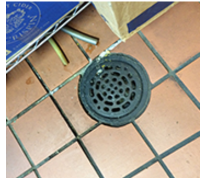
Eroded grout at drain.
