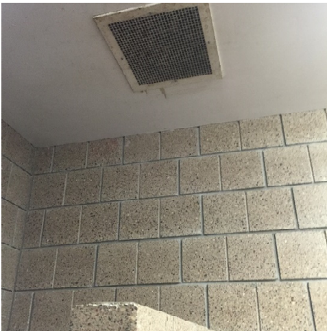
Restroom exhaust grille.
