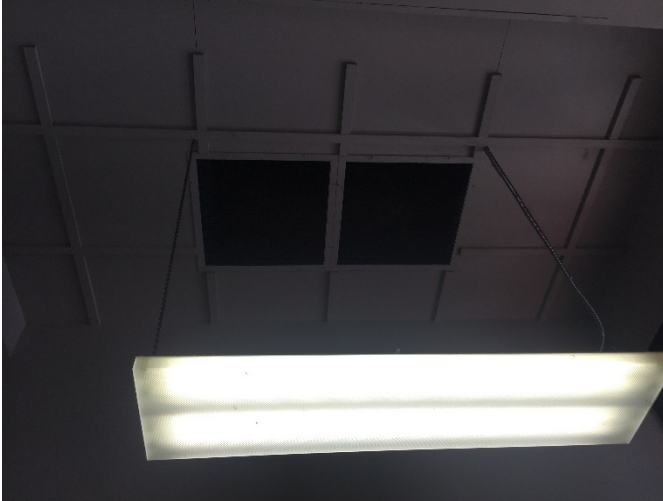
Makeup air intake grilles.
