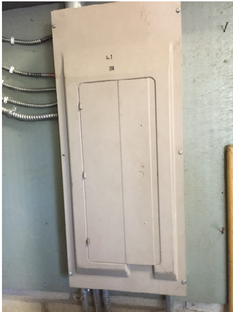
(2) 200A panels are in fair condition.
