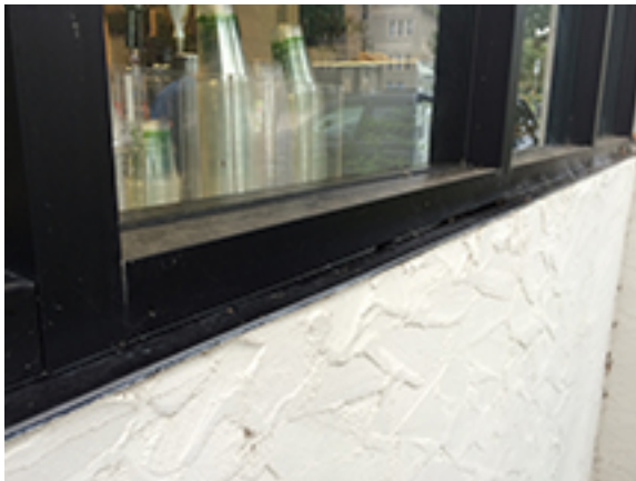
Water collecting at sill flashing.
