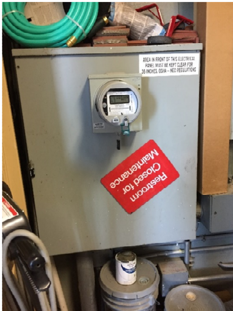
Incoming Xcel service.
