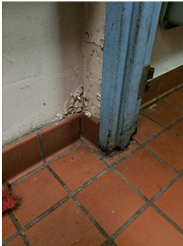
Bottom of wall.
