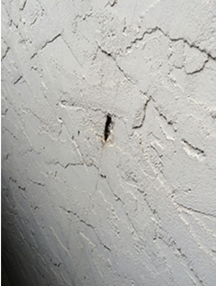
Damage to Stucco Finish.
