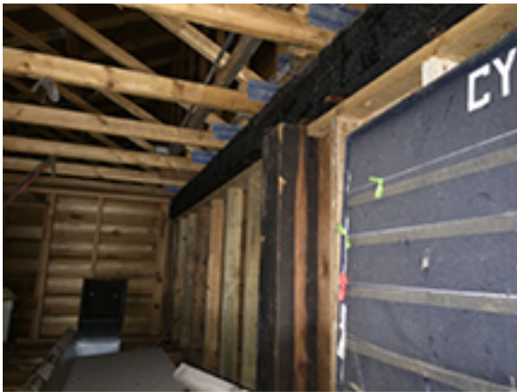
Fire damage at roof structure.
