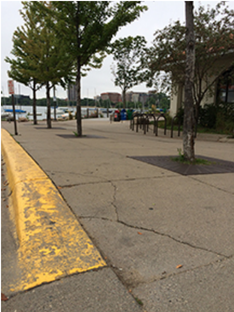
Cracking at drop-off.
